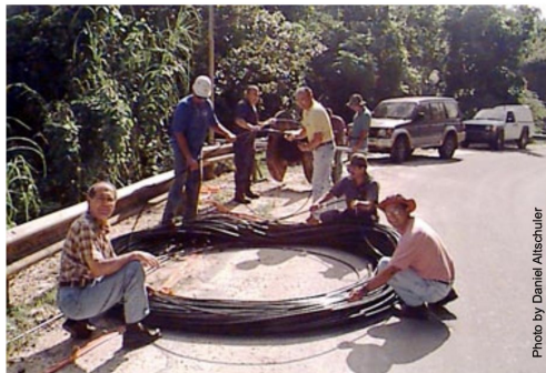
Observatory electronics and maintenance personnel installing fiber optic cable for T1 internet and telephone service.
